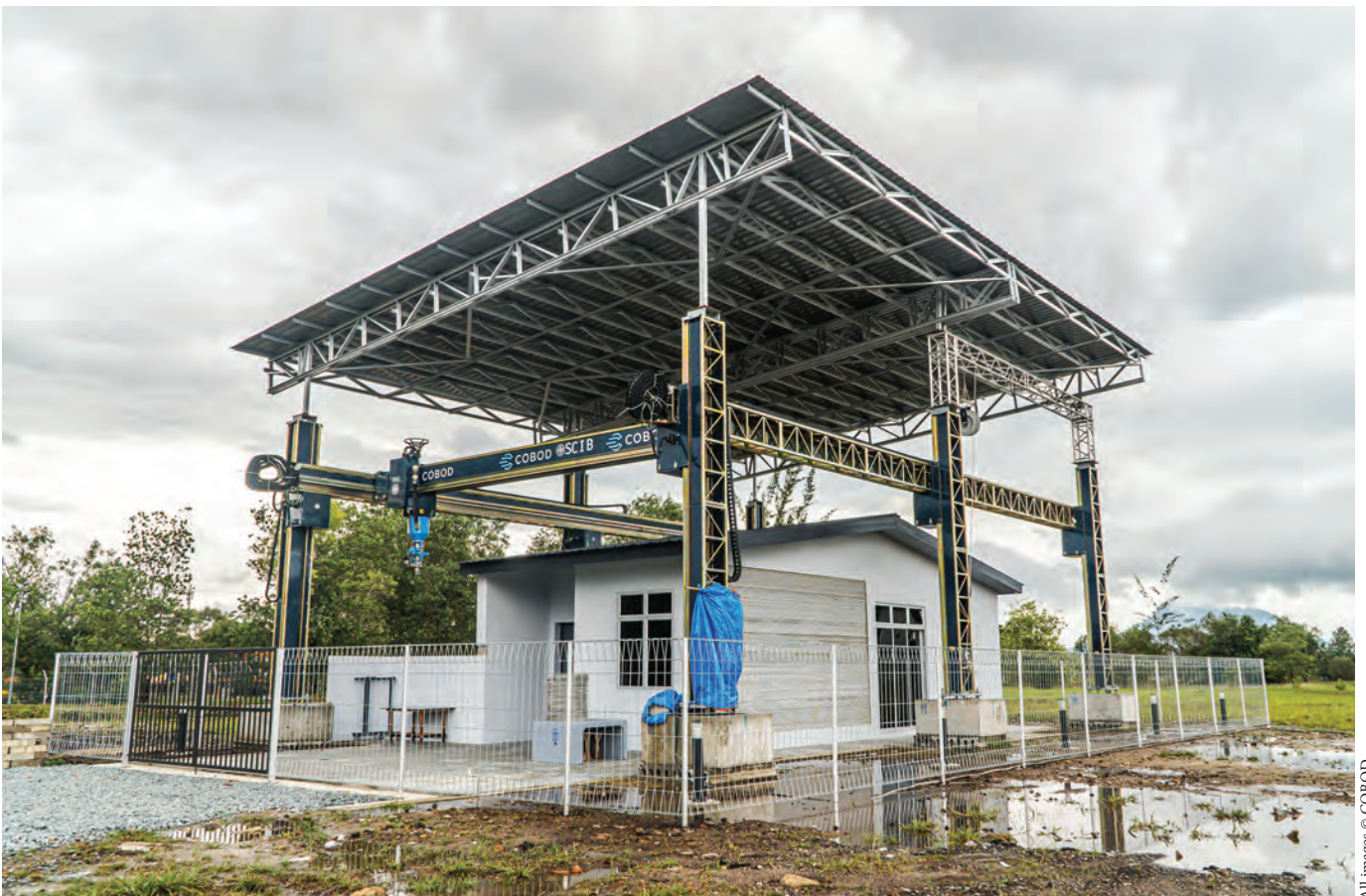
TOP: Due to high-humidity weather conditions in the region, the SCIB team chose to plaster the outside walls of the house. OPPOSITE AND ABOVE: The total printing time for the house was 46 hours, using a BOD2 3D construction printer from COBOD.
