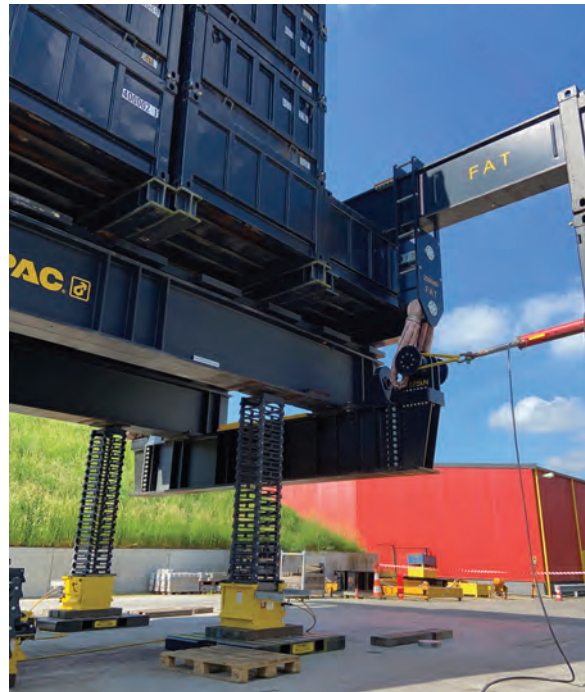
LEFT AND BOTTOM LEFT: Four Enerpac SCJ-100 Cube Jacks lift a 400-t load during testing.
