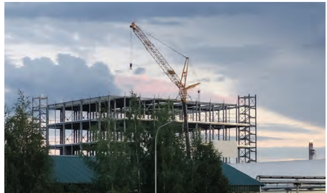
In another project, MyCrane has provided independent advice for a global energy customer that needed to install nine pieces of equipment.
